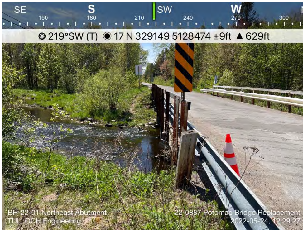
Photo 2: View from Drill Rig set up at BH-22-01 and view of the east side of the existing bridge
