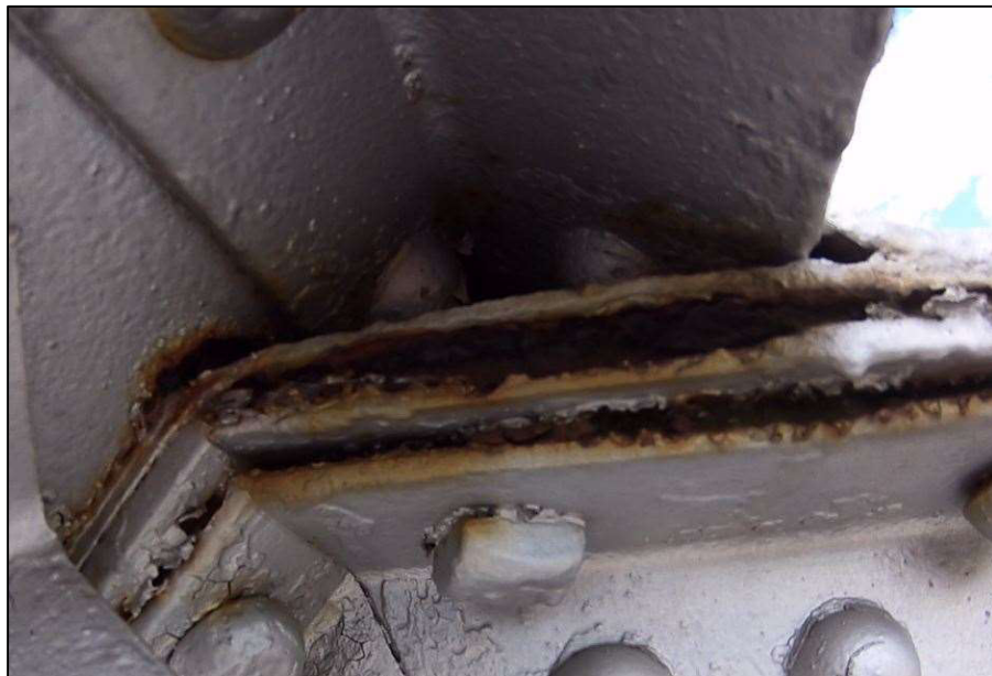
Figure 10 - Typical Rust Jacking at Upper Truss Connections
