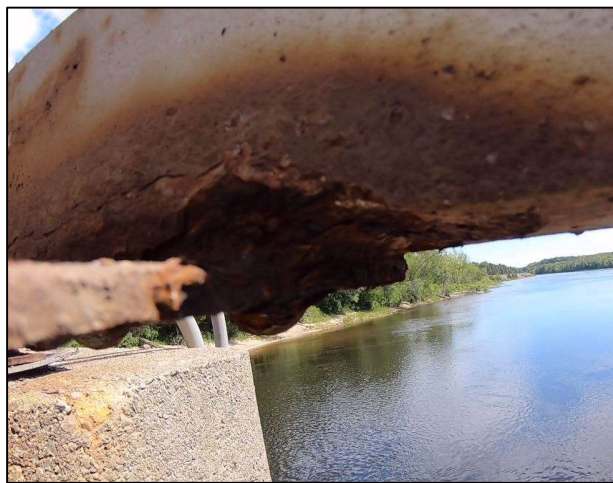
Figure 2 - Severe Section Loss in Bottom Chord
