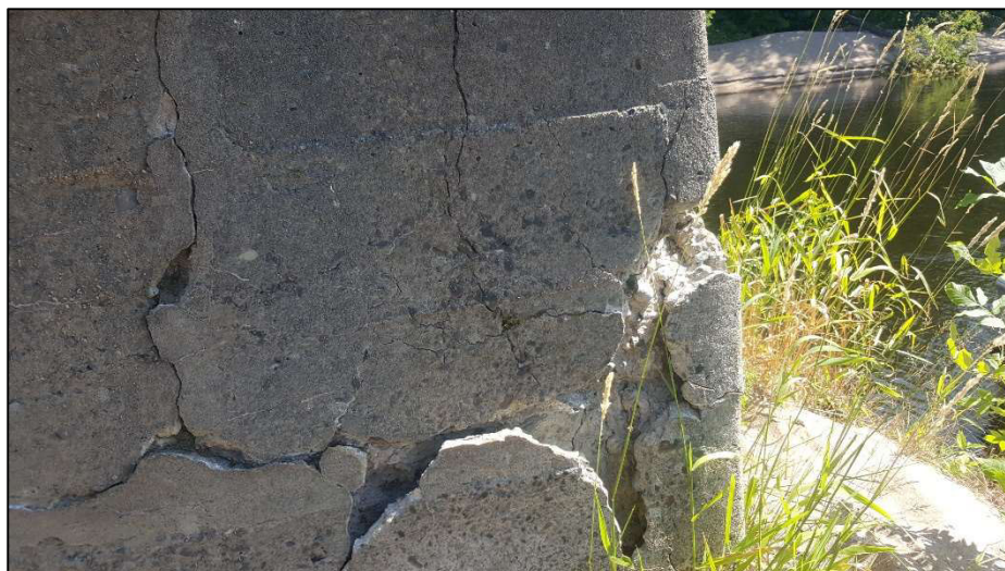
Figure 16 - Wide Crack and Severe Delamination at Bottom of South Intermediate Pier
