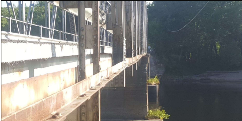
Figure 13 - Deflection in Bottom Chord (South Span)
