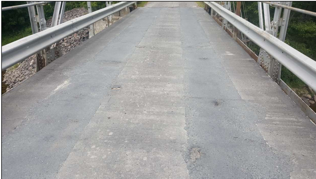
Figure 5 - Typical Wearing Surface on North Span (Patching of the 1 st installed deck panel)
