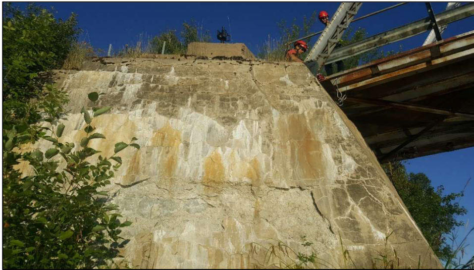
Figure 17 - Wide Cracks, Spalls, Delamination and Efflorescence and Map Cracking in Concrete Abutment/Wingwall
