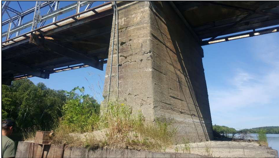
Figure 15 - Spalls, Cracking and Efflorescence at South Intermediate Pier
