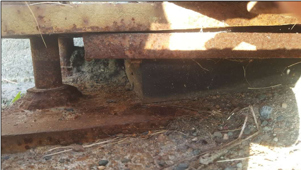
Figure 14 - Gravel Buildup on Bearing Pad
