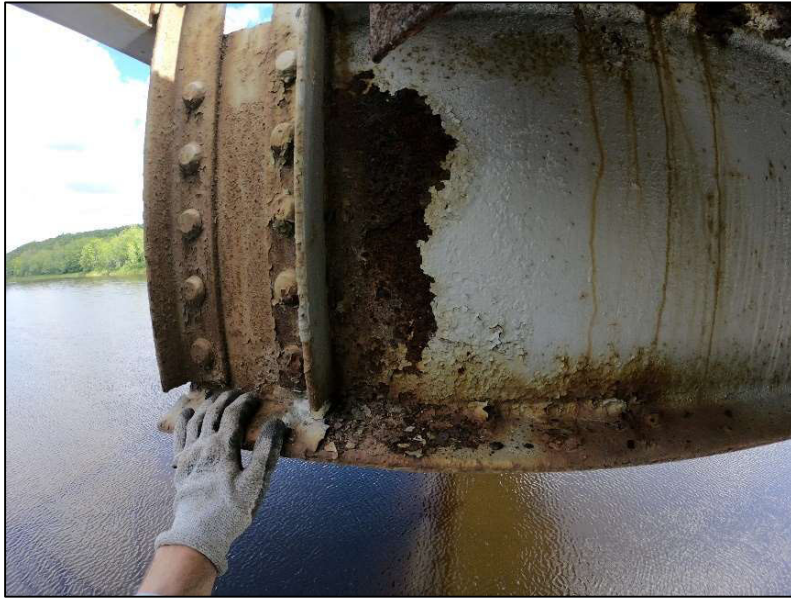
Figure 9 - Typical Floor Beam Connection/Flaking of Protective Coating
