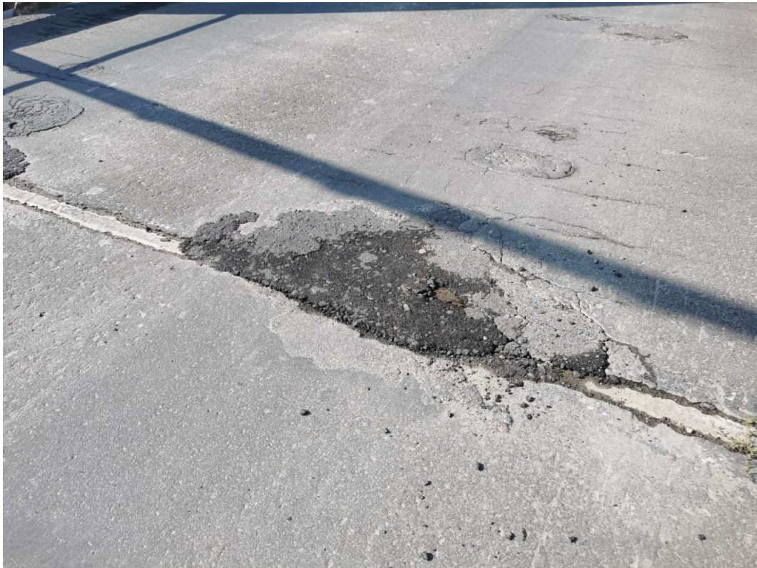
Large Potholes, De-bonding and Transverse Cracking in Overlay
