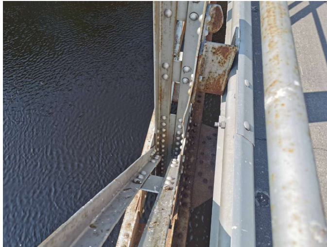
Hand railing with breakdown of protective coating
