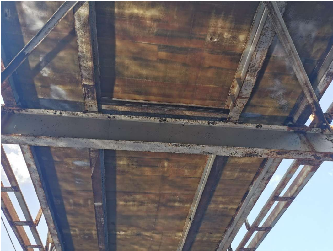
Staining of Floor Beams at Edges of Deck (staining below shim plates under exterior stringers)
