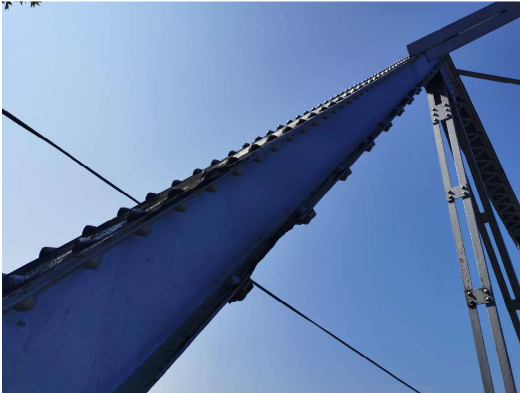
Top Chord - Built up Box Section. Various locations with impact damage to the interior edges.
