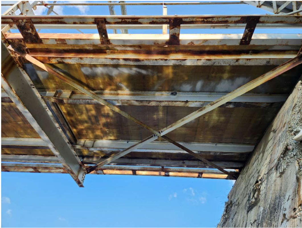
Typical Protective Coating Condition
