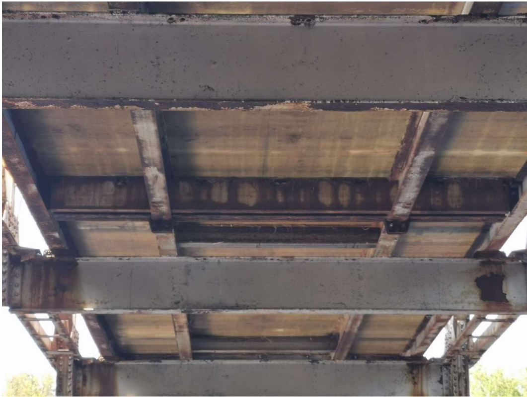
Typical Floor Beam - Pitting and Flaking Present on End Sections
