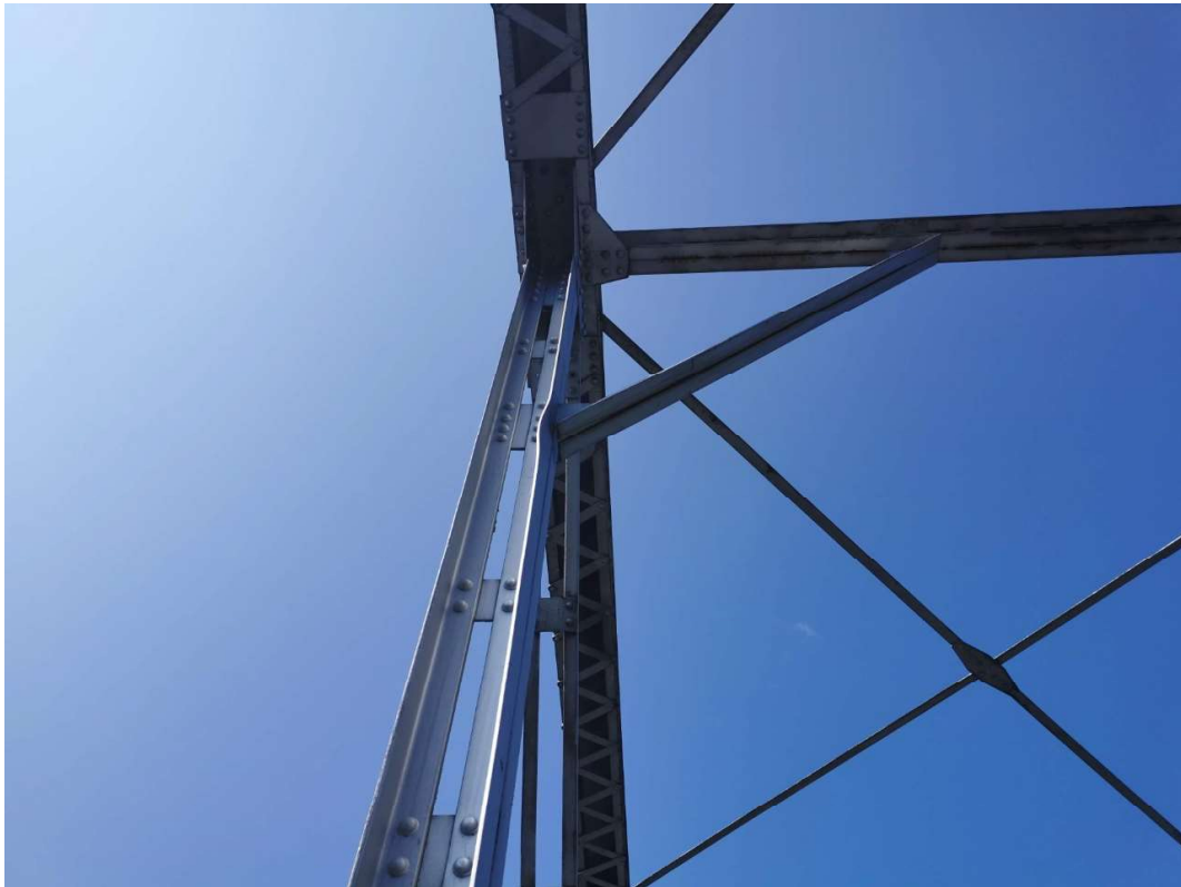
Warping of Vertical near connection to 'K' bracing
