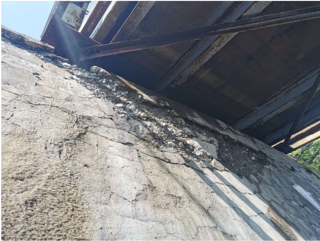
Severe Spalling, Delamination and Efflorescence Throughout Abutment Walls
