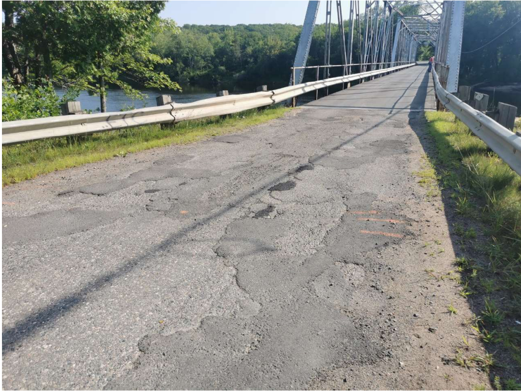
Patches and Potholes in South Approach
