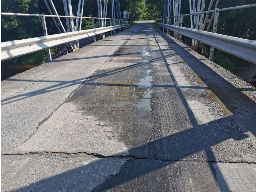
Patches, Wheel Rutting and Ponding Water on North Span
