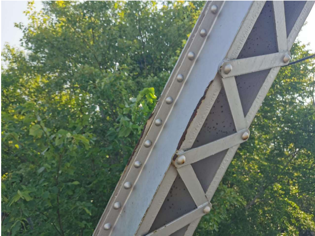
Impact damage to inner surface of the top chord (~3.5m above bridge deck)
