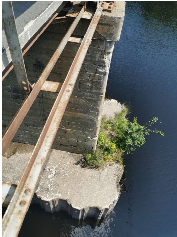
Typical Pier With Localized Spalling and Medium to Wide Cracking Throughout
