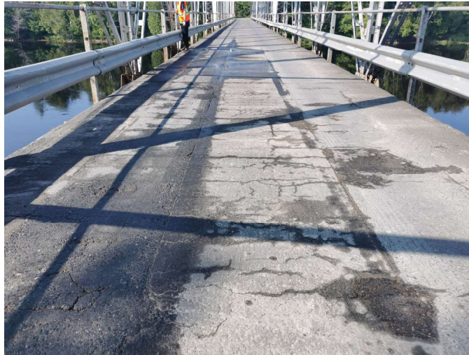
Breakdown of Coating throughout railing/posts.
