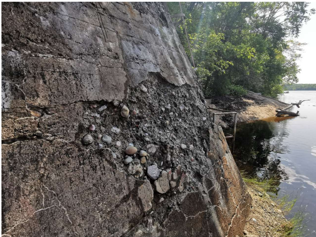
Severe spalling, delamination and map cracking with efflorescence (north abutment worse)
