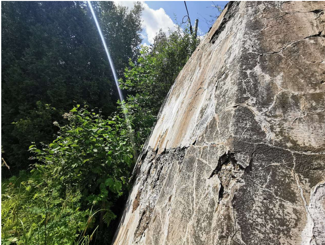
Delaminations and Efflorescence Throughout Wingwalls
