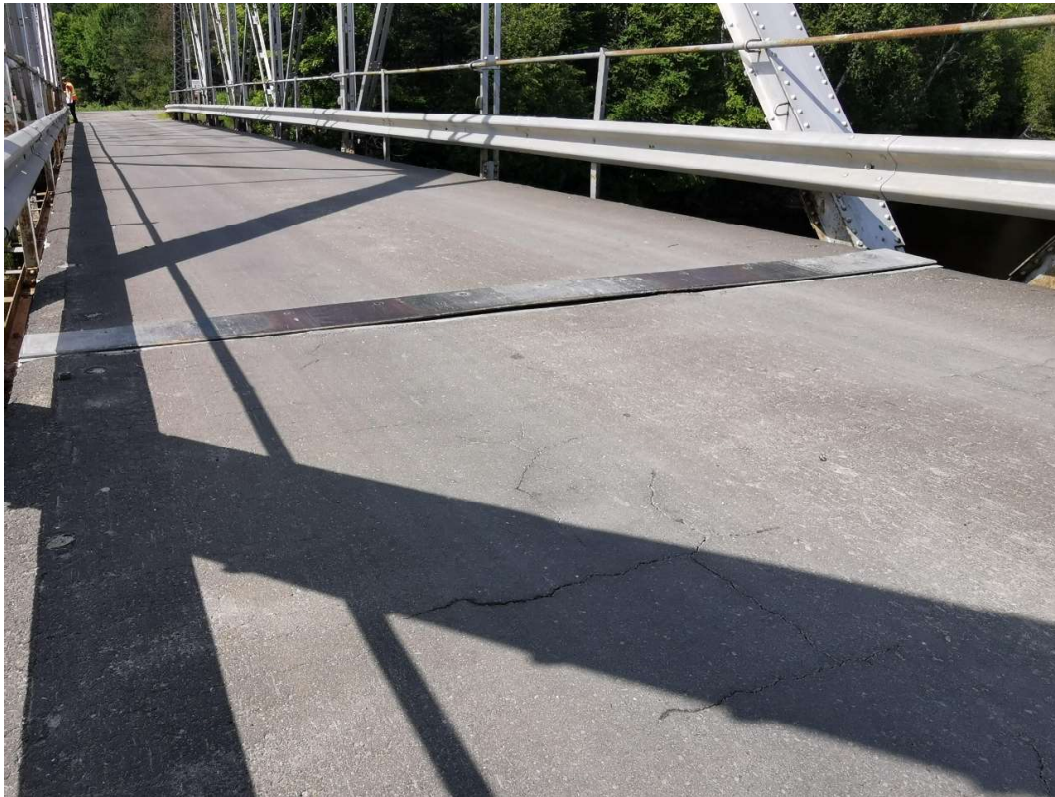
Lifted Armouring Plate at Centerline, Rotated at West side of Bridge
