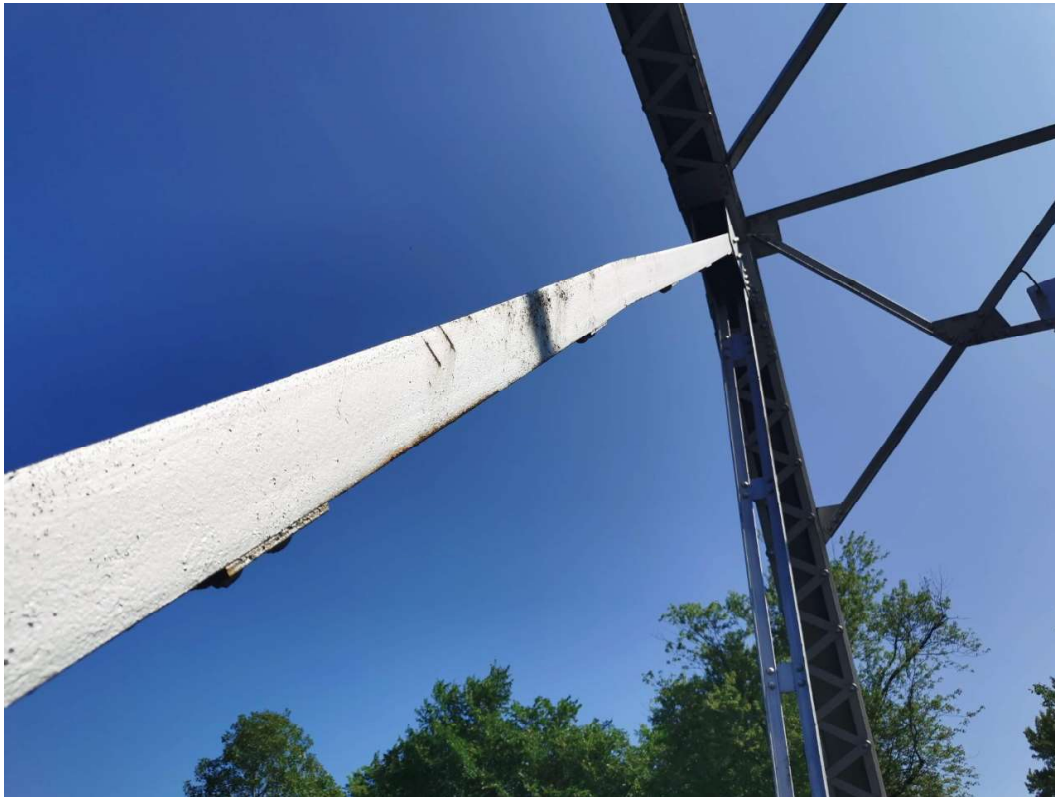
Localized distortion of diagonal (inner) on the West Truss at North Abutment
