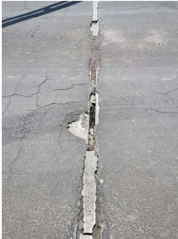
Joint Seal Severely Deteriorated with Sections Missing
