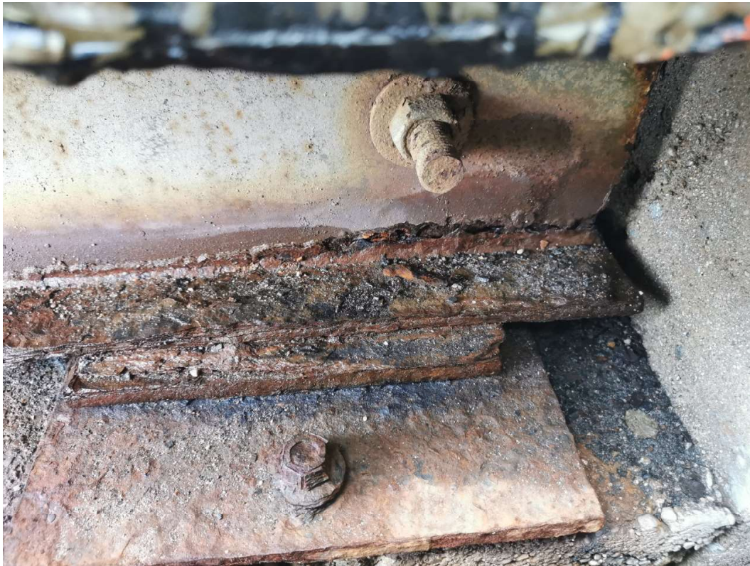
Localized Severe Corrosion and Cracking in Web of Exterior Stringer at North Abutment
