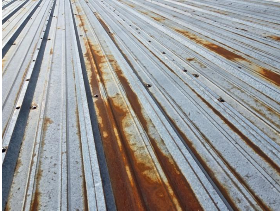
Figure 5: Corroded roof section
