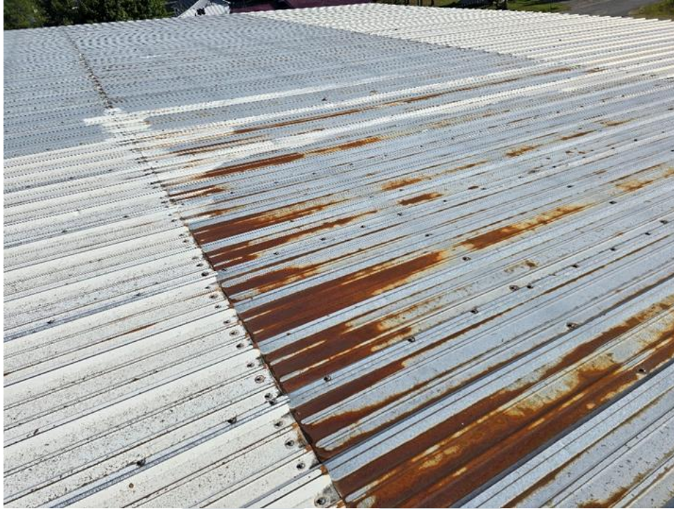
Figure 3: Corroded roof section
