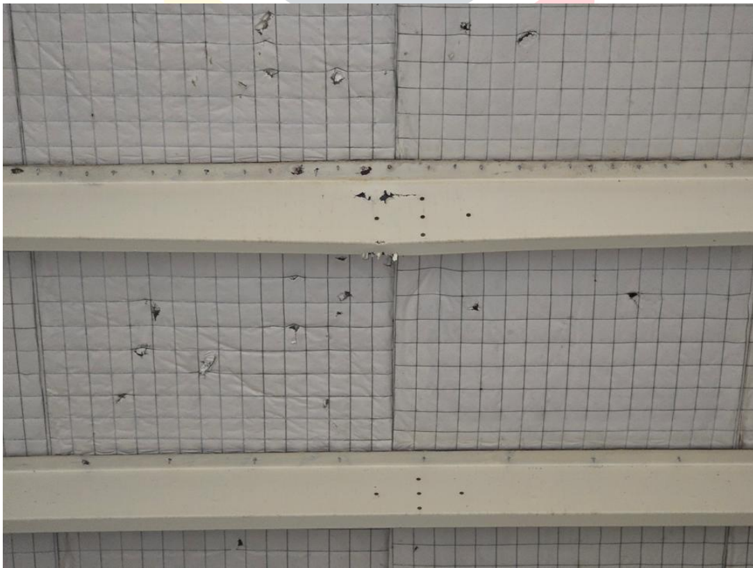
Figure 6: Bent roof purlin
