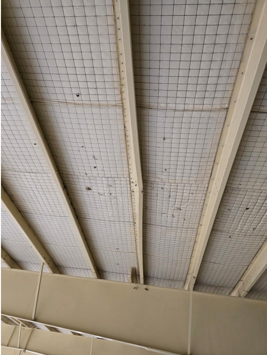
Figure 7: Bent roof purlin
